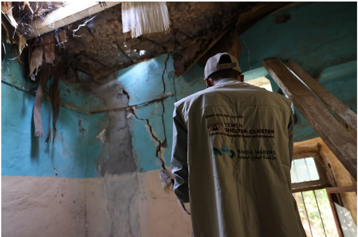
Fig 11-20 NMO engineer conducts a thorough assessment in a damaged room in Salah, Taiz. The visible deterioration of the ceiling and walls underscores the severe impact of armed conflict, highlighting the critical need for intervention and support from the shelter cluster.
