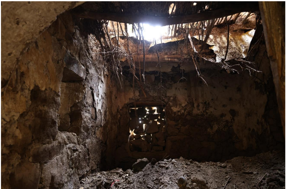
Fig 11-6 Inside another room of the abandoned house in Saber Al Mawadim, sunlight filters through the crumbling roof and a broken window, casting eerie shadows on the walls and revealing the remnants of a once-vibrant space now overtaken by nature.
