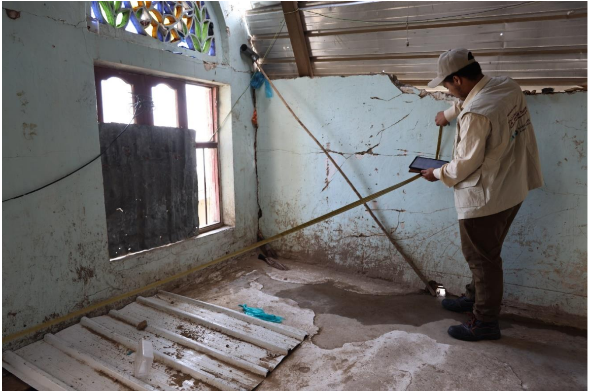
Fig 11-9 NMO engineer conducts a technical assessment of a damaged room in a house in Saber Al Mawadim, Taiz, which has become uninhabitable due to war. While the house owner resides in a safer area of the home, this section is no longer suitable for living.
