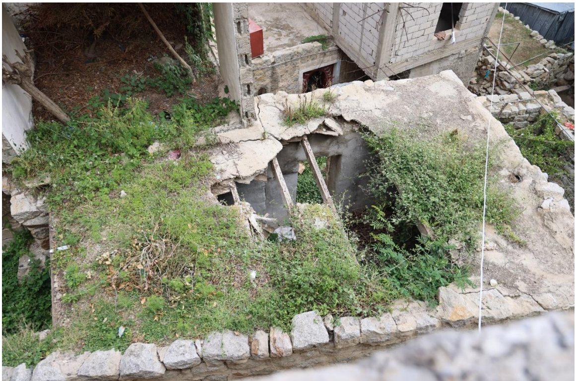
Fig 11-10 An overview of a deteriorating structure in Saber Al Mawadim, Taiz, where nature is reclaiming the space. The roof has collapsed, and vegetation now flourishes in the once-occupied area, highlighting the impact of abandonment and the effects of war.
