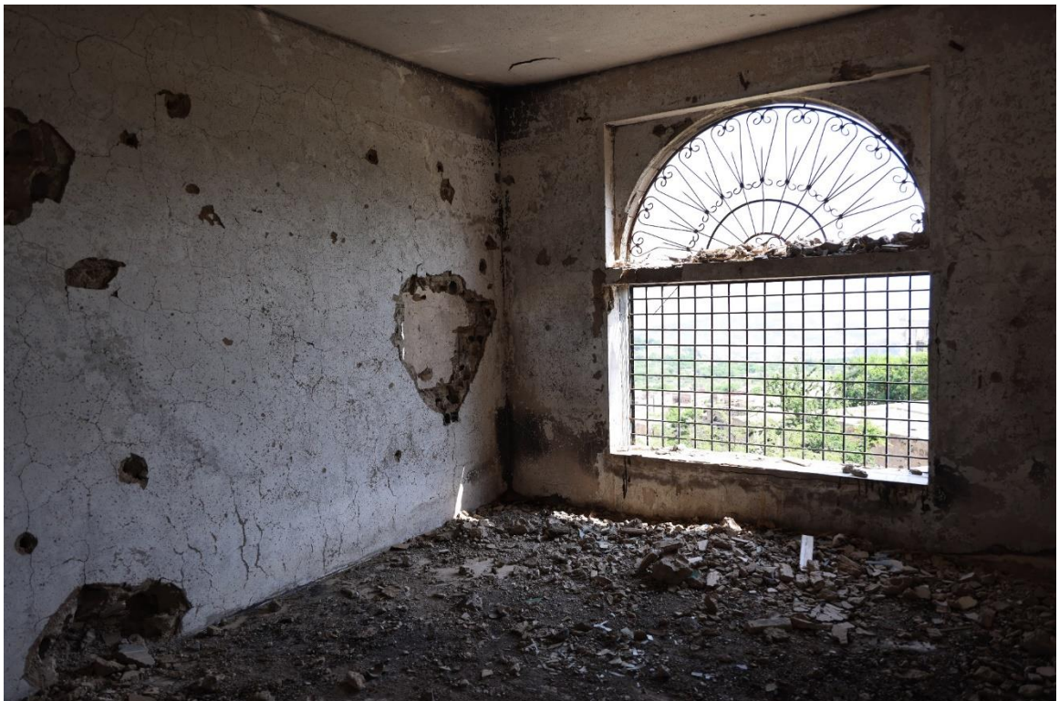
Fig 11-18 Inside another damaged room in Salah, Taiz, the walls bear the scars of conflict with visible cracks and debris scattered across the floor. The light filtering through the broken window highlights the extent of neglect and the urgent need for restoration.
