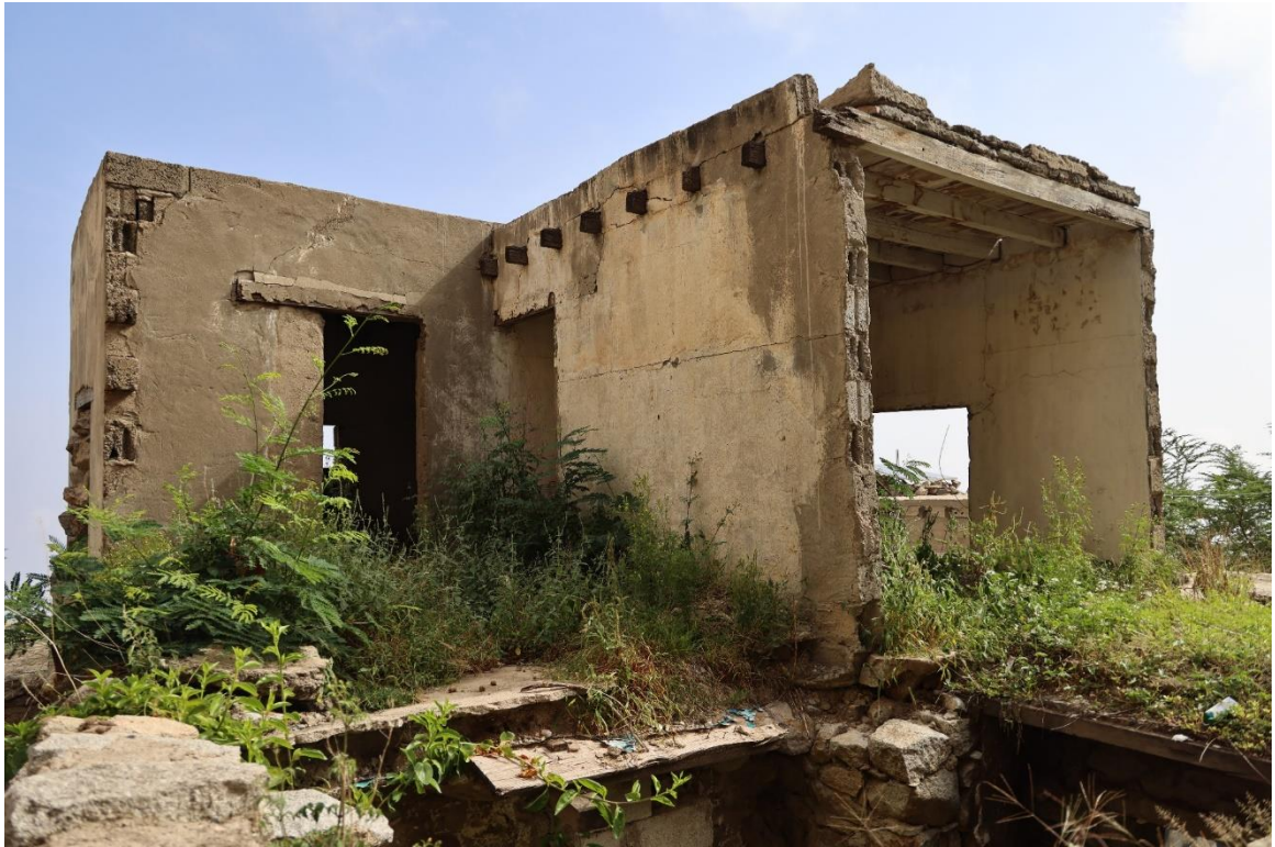
Fig 11-13 Remnants of a building in Saber Al Mawadim, Taiz, stand in stark contrast to the encroaching vegetation. The structure, abandoned and damaged by the war, reveals open doorways and collapsed sections, symbolizing the ongoing impact of conflict on the community.
