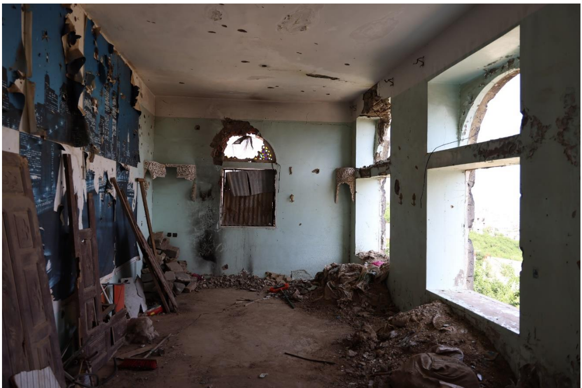
Fig 11-16 Inside a damaged room in a building in Salah, Taiz, remnants of wallpaper and broken windows reflect the destruction wrought by war. The debris scattered across the floor and the exposed walls tell a story of neglect and the urgent need for reconstruction.
