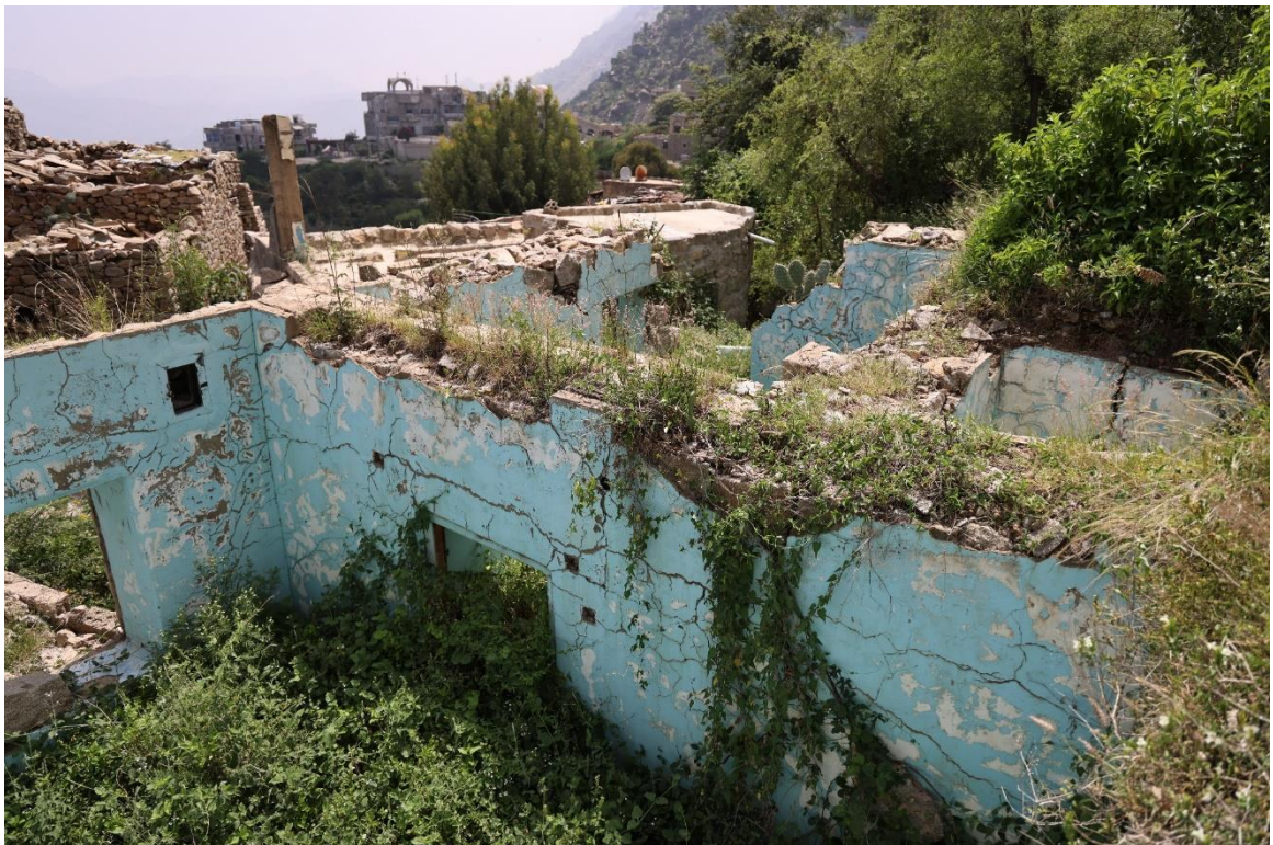
Fig 11-2 Fully damaged houses in Saber Al Mawadim, Taiz, overgrown with vegetation and deemed unsuitable for living.
