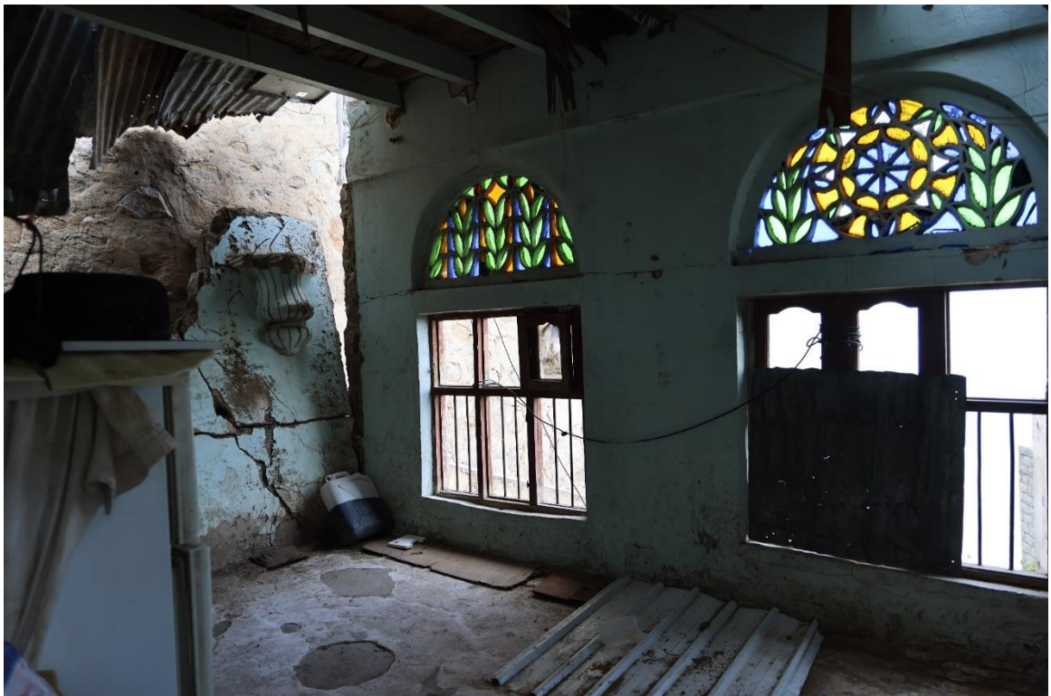
Fig 11-12 Inside a once vibrant room in Saber Al Mawadim, Taiz, the remnants of stained glass windows and cracked walls tell the story of a home damaged by armed clashes during the war. The side wall has collapsed, leaning precariously against the nearby mountain.
