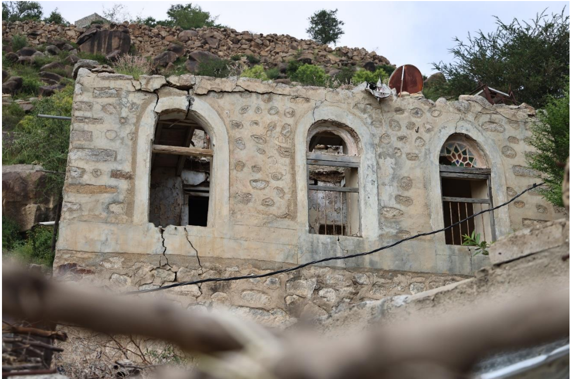
Fig 11-11 Cracked and weathered, the facade of an abandoned house in Saber Al Mawadim, Taiz, reflects the toll of conflict. The remnants of its architectural beauty stand in stark contrast to the neglect and devastation surrounding it.
