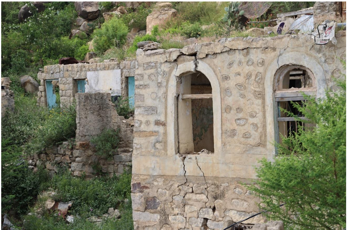
Fig 11-8 Remnants of an old home in Saber Al Mawadim, with cracked walls and broken windows, stand as a testament to the destruction wrought by war, now overrun by nature and time.
