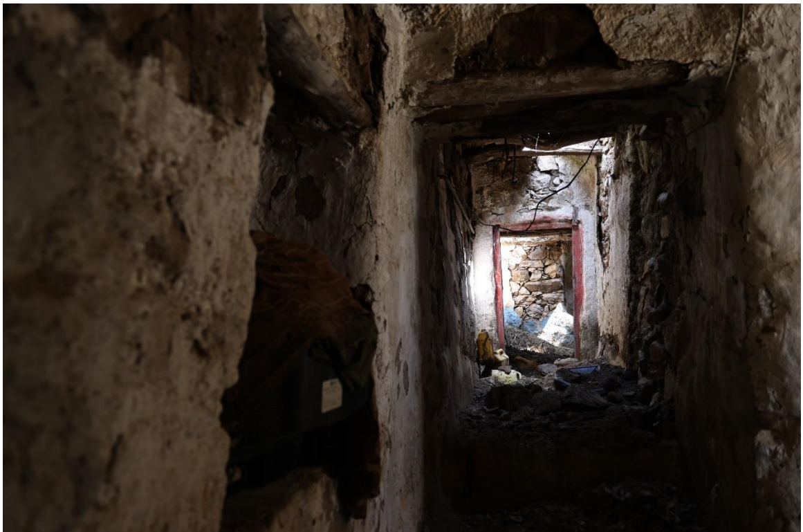
Fig 11-4 An abandoned old house in Saber Al Mawadim, left by its owners due to the impact of war, now stands in disrepair and is unsuitable for living.
