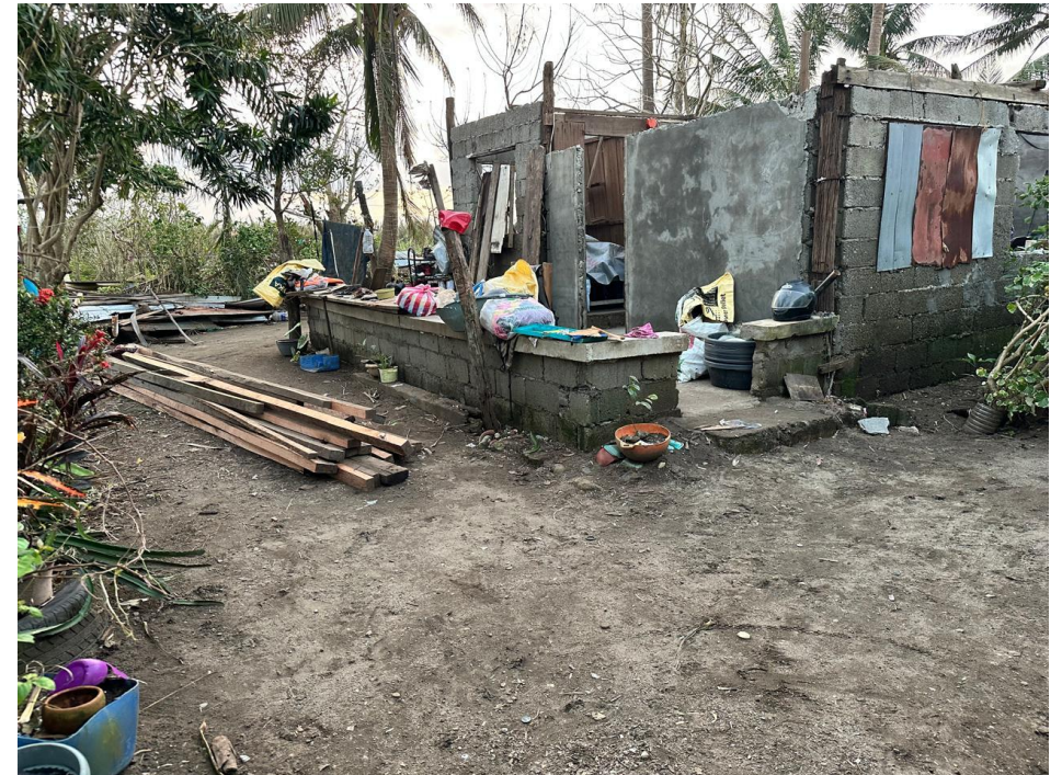
A damaged house in Santa Ana, Cagayan where Typhoon Marce (Yinling) first made landfall. © WFP/Nicole Pagulong
