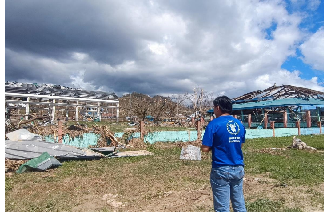
WFP staff surveys the infrastructure damage caused by STY Pepito in Dipaculao, Aurora. © WFP/Arlene Robles
