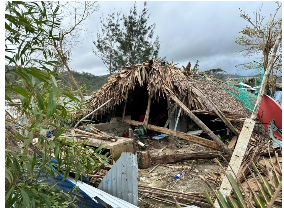
A collapsed house in Claveria, Cagayan where one casualty was recorded following the onslaught of Typhoon Marce (Yinling). © WFP/Nicole Pagulong
