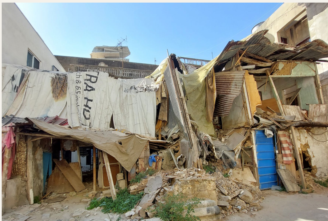
A fragile structure severely damaged after the Beirut blast. September 2021 Source: Abir Zaatari/American University of Beirut
