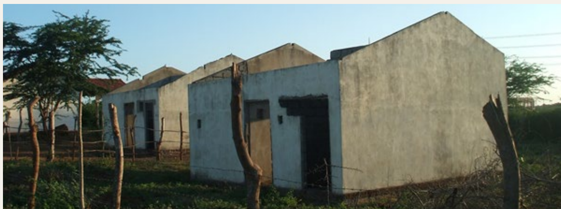
Abandoned and vandalised houses in Hambantota-New Town, Sri Lanka Source: Dr Iftekhar Ahmed
