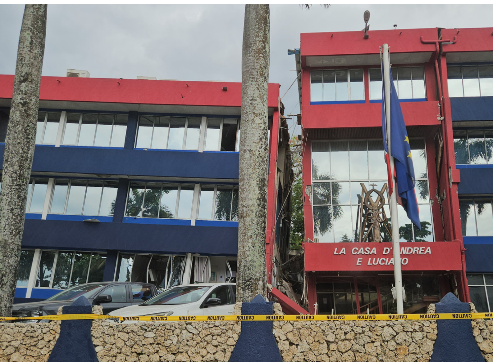
Picture 4: Building damaged
