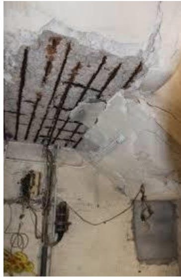
Deterioration of Concrete
