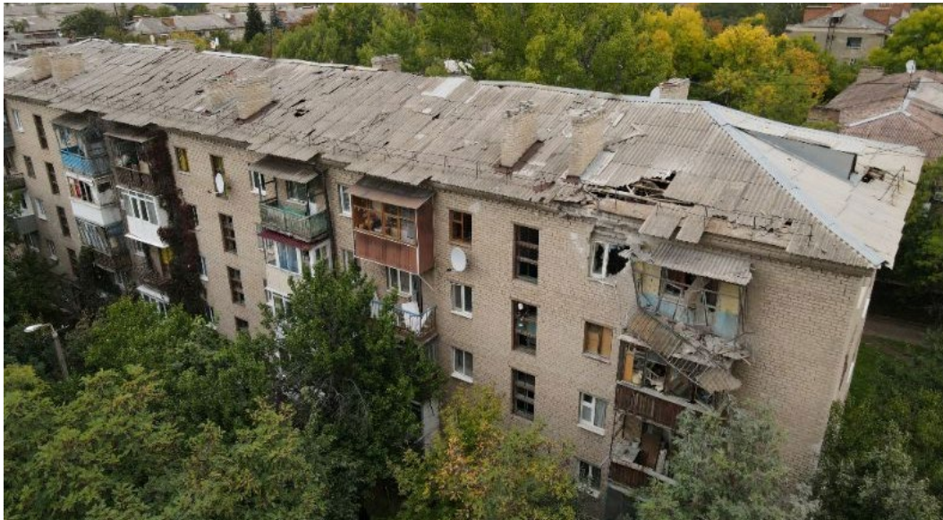
Figure 2 – The damaged hipped (non-flat) roof of the multi-storey building, Kramatorsk, credit https://www.kramatorskpost.com/
