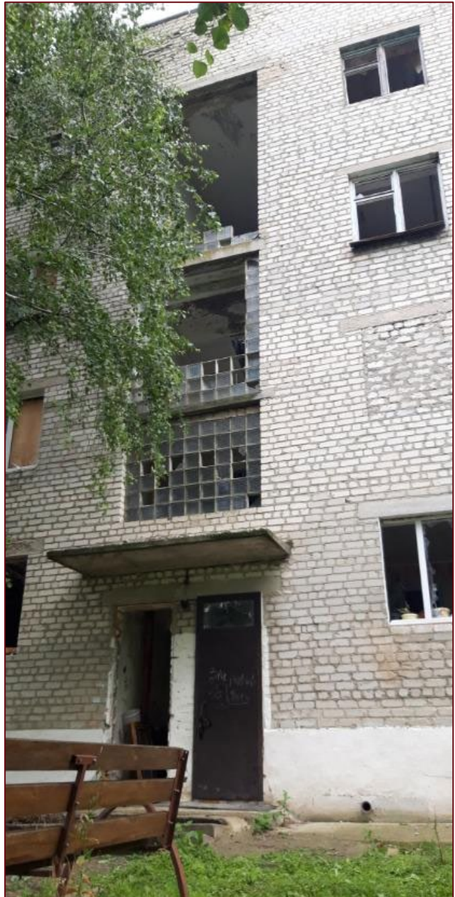
Figure 4 – Damaged windows in common space, Kharkivska oblast, credit https://dream.gov.ua/
