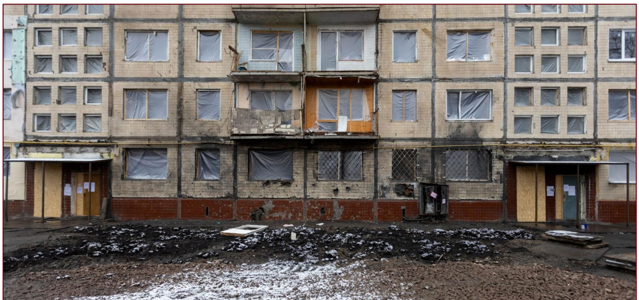
Figure 5 – Damaged windows and external doors of entrance group, Kyiv, credit https://rubryka.com/
