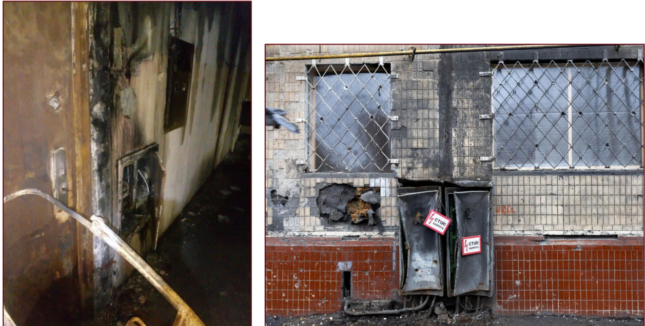
Figure 6 - Electrical panels with clear signs of heat and fire damage, multi-apartment buildings, Kharkiv (left), credit https://dream.gov.ua/ , Kyiv (right), Photo by Mykola Tymchenko (credit https://rubryka.com/ )
