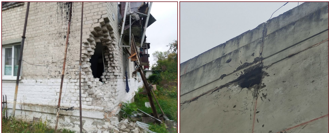
Figure 7 – The damage caused by the direct strike of a projectile, such as shell fragments or debris from an explosion, Pokrovske (left) and Kharkiv (right), credit https://dream.gov.ua/
