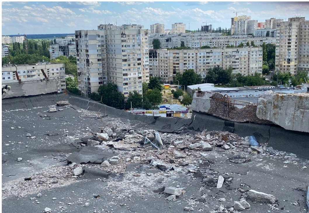
Figure 3 – The damaged flat roof of the multi-storey building (with partial destruction of parapet), Kharkiv, credit https://dream.gov.ua/
