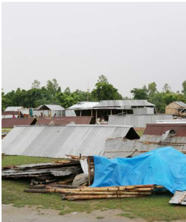
Household damaged by storm
