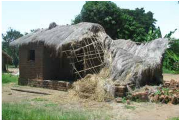
11. House collapsed because of the earthquake
