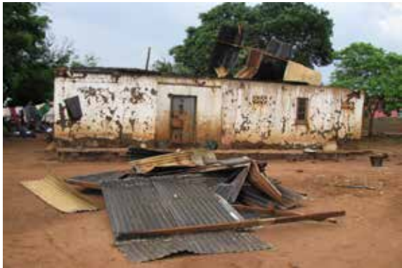
10. Blown off roof
