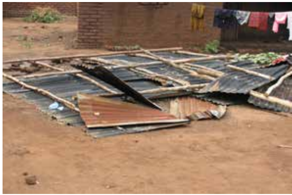
9. Blown off roof
