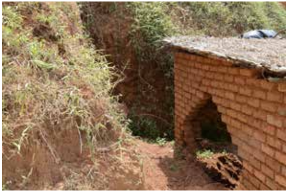
14. Wall collapse after landslide
