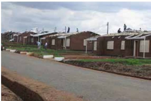
16. Blown off roof
