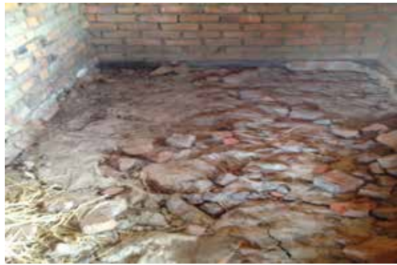
2. Mud pavement erosion due to water exposition
