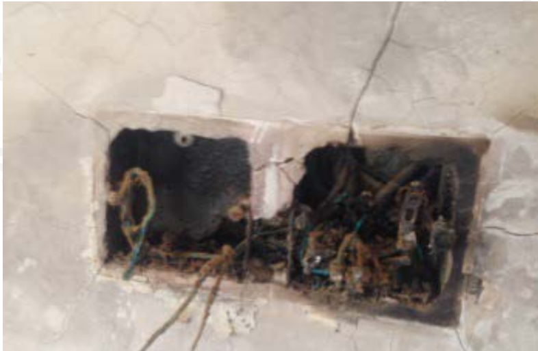
Unsafe conditions in critical shelters: Communities were living with exposed electrical cables, which made them highly vulnerable to electrocution.
