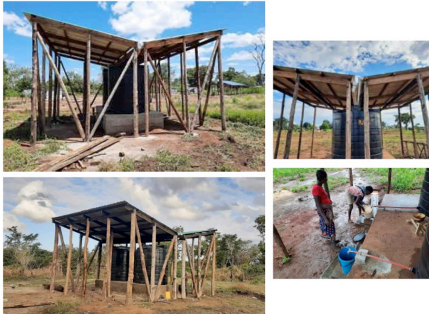
Rainwater Harvesting facilities
