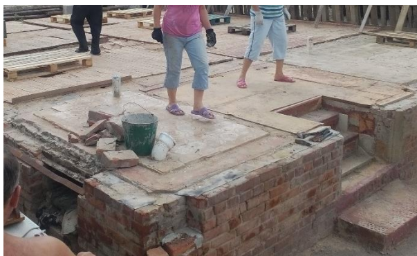
Figure 20 Some houses have floors which are fully reusable especially those made from non-flammable material as ceramic floor tiles. (ADRA project Slovyansk 2015).
