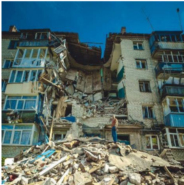
Figure 9 A large calibre strike brought down several floors, even if the structural integrity of the building was seriously affected, both sides are still useable.
