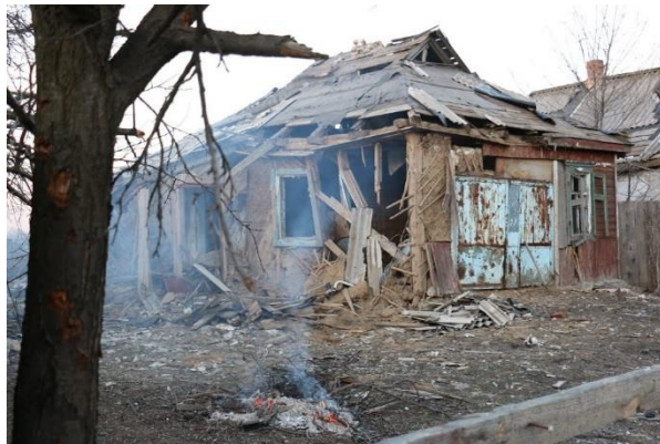
Figure 35 Damaged wattle & daub house. People in Need assessment in Nikishine, 2015. Credit R. Lunin
