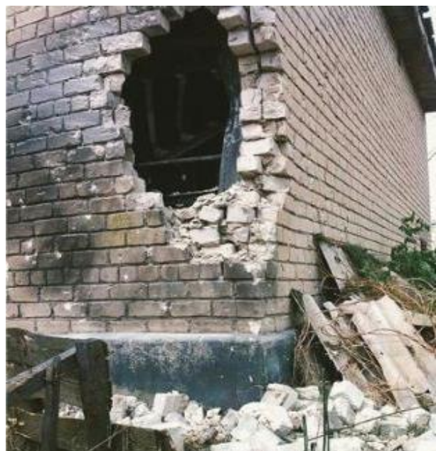
Figure 7 Small calibre direct hit, repairable with adequate techniques
