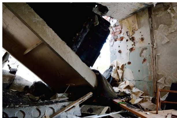
Figure 11 Inside an apartment after shelling, People in Need assessment, 2015. Credit R Lunin
