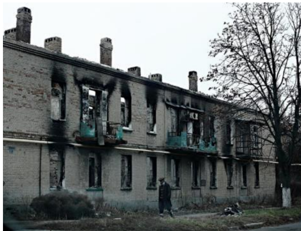
Figure 8 Results of fire damage to brick building.
